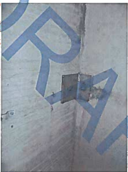
Figure 42: Steel Connector in Near to Original Condition
