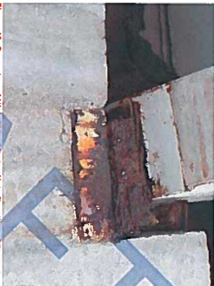
Figure 46- Corrosion of High Shim Stack - Note Rotation of Precast Beam
