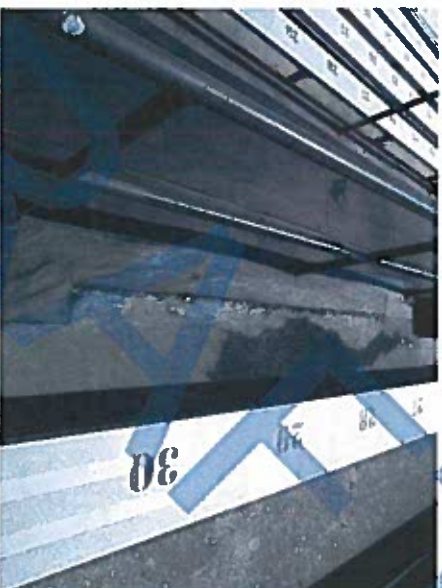
Figure 40- View of Delaminated Membrane
