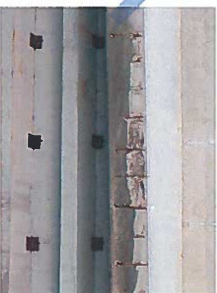
Figure 56 - Concrete Spalling at Main Frame Beam
