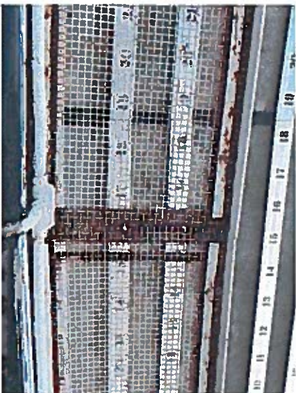
Figure 83- Corrosion of Steel Mesh Sunscreen
