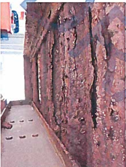
Figure 73 - Severe Corrosion of Steel and Deck at Bridge Stair
