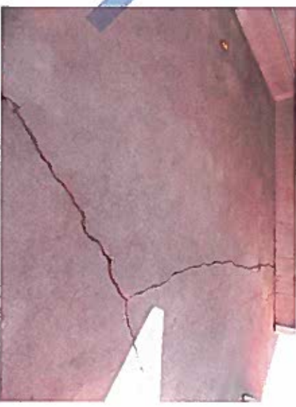
Figure 69- Frost Heave at Slab on Grade in Concessions
