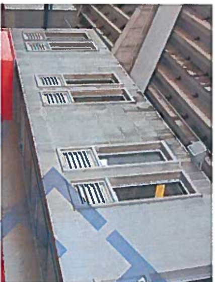
Figure 27- Mezzanine Exterior Wall- Staining
