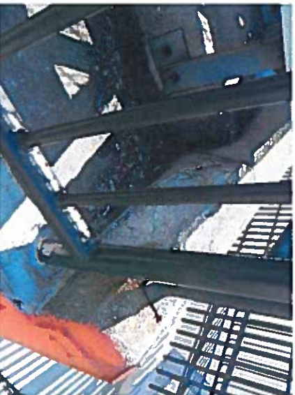
Figure 62- Deterioration of Concrete Retaining Wall
