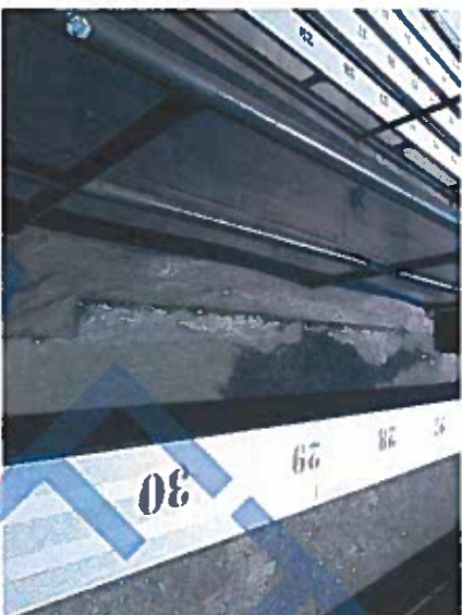
Figure 54- Waterproofing Membrane at Precast Top - Failure
