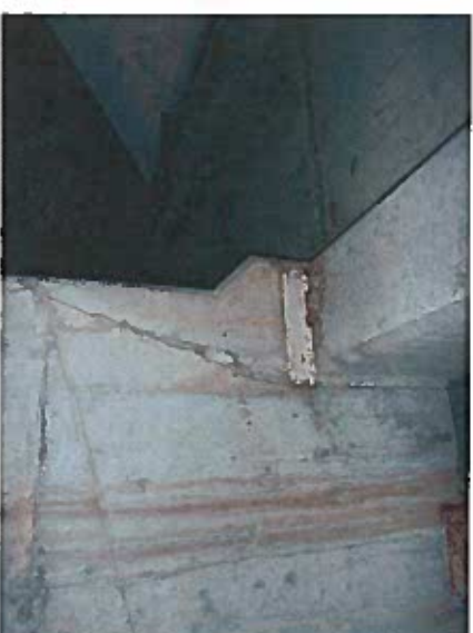
Figure 61- Cracking and Failure of Corbel
