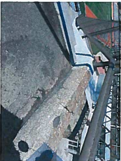
Figure 58- Deterioration of Slab and Curb
