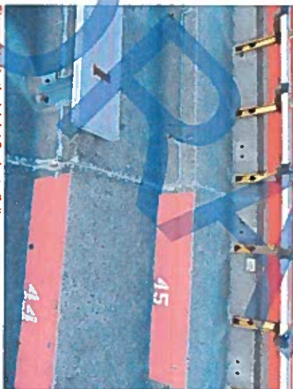
Figure 51- Vertical Joint Sealant - Failure
