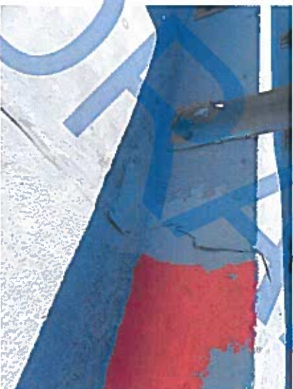
Figure 55- Applied Traffic Coating - Failure at Joint
