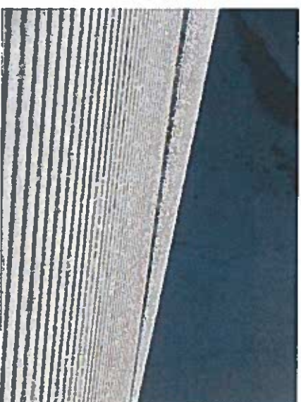
Figure 79 - Bulge in Precast Panel
