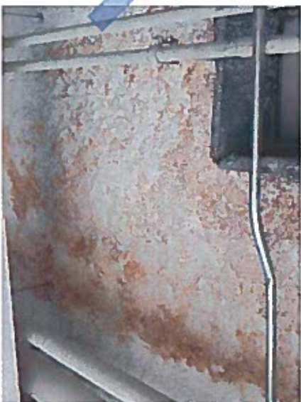
Figure 82 - Mold/Discoloration of Spray on Insulation
