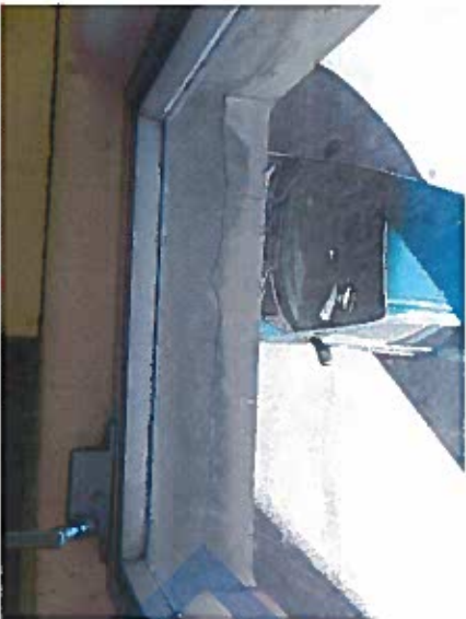
Figure 80- Crack in Precast Window Surround
