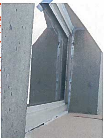
Figure 78- Window Sealant Joint - Deteriorated
