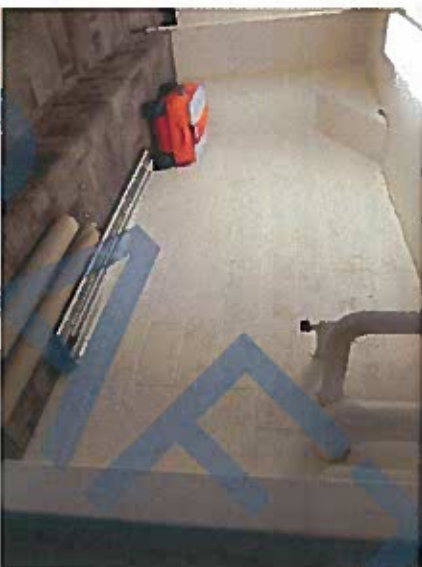
Figure 77: Moisture Penetrating into CMU Wall From Above
