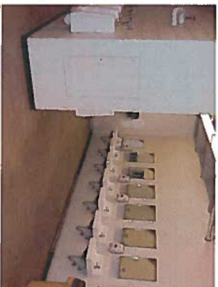
Figure 9- Public Toilets- Lavs
