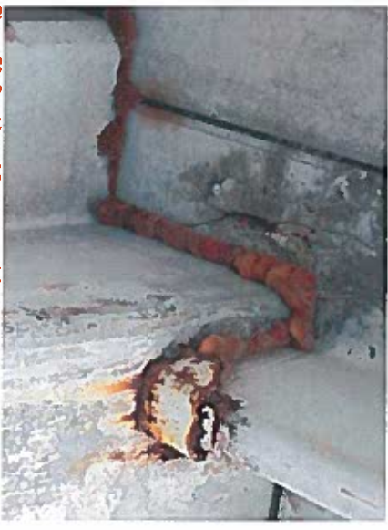
Figure 70- Cracking of Concrete and Corrosion of Steel Embeds
