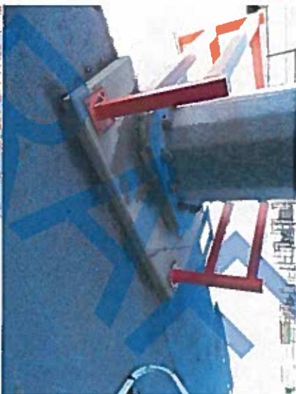
Figure 68- Light Pole Support Base Cracking and Grout Deterioration
