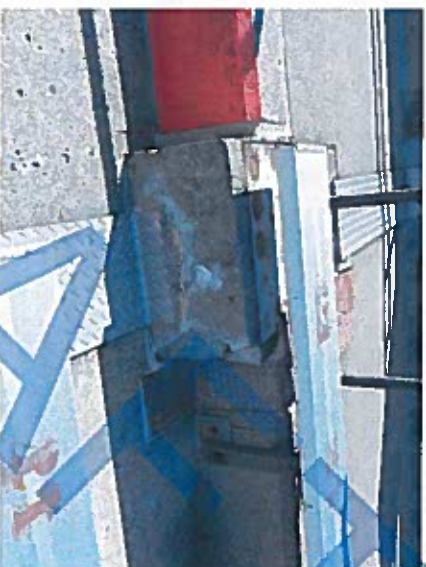
Figure 59- Deterioration of Exposed Concrete Column at Embed Plate
