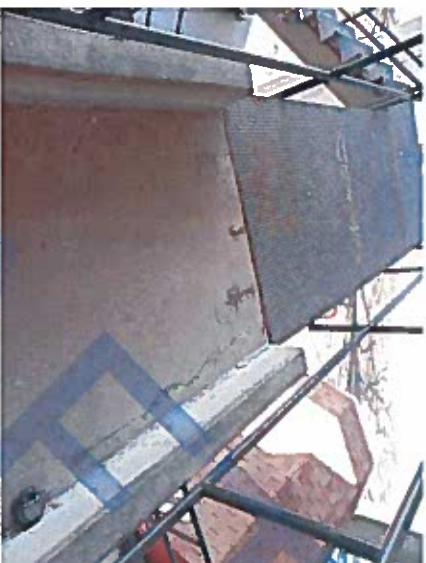
Figure 72 - Minor Corrosion of Checkered Plate Stair
