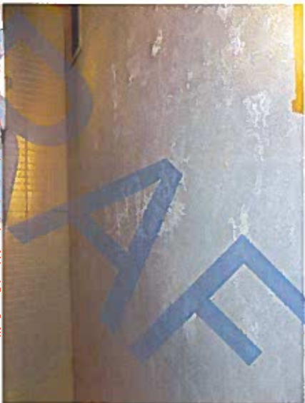
Figure 81- Humidity Corroding Under side of Hard Pan Ceiling
