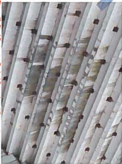
Figure 43: Steel Connector Typical Corrosion of Exposed connectors
