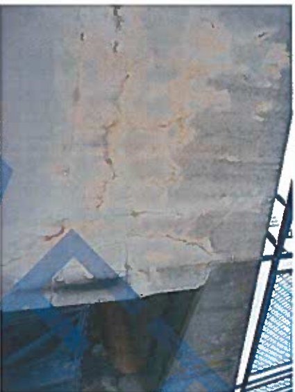
Figure 63- Deterioration of Concrete Retaining Walls
