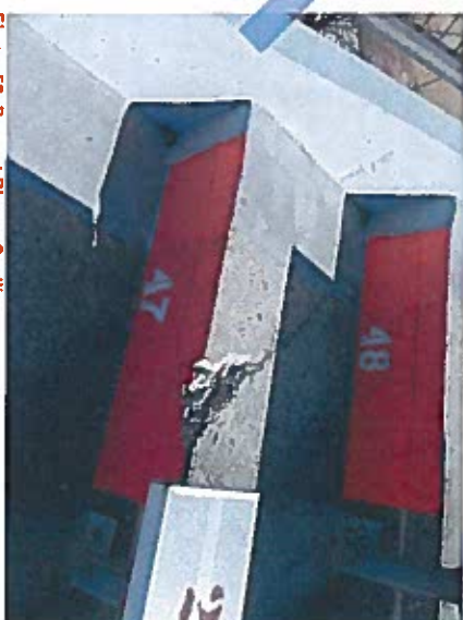
Figure 52- Precast Riser - Spalling
