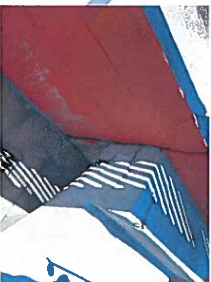
Figure 65- Deterioration of Concrete Stair and Wall
