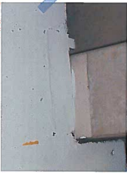
Figure 47- No Corrosion at Expansion Joint - No Welds
