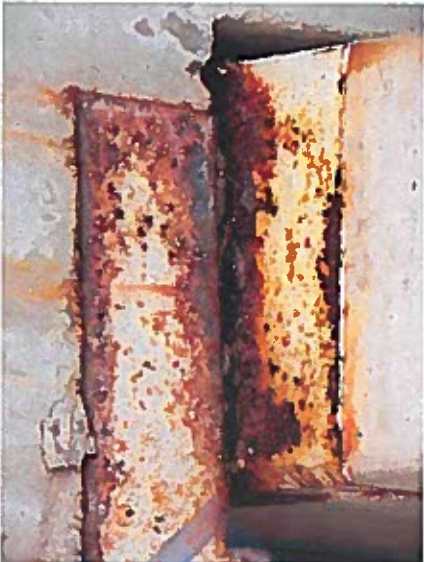
Figure 45- Corrosion at Thin Shim Plate - Welded completed Deteriorated
