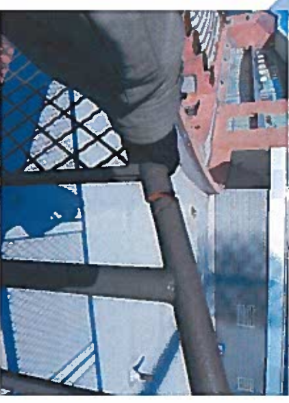
Figure 74 - Split in Guardrail Top Rail
