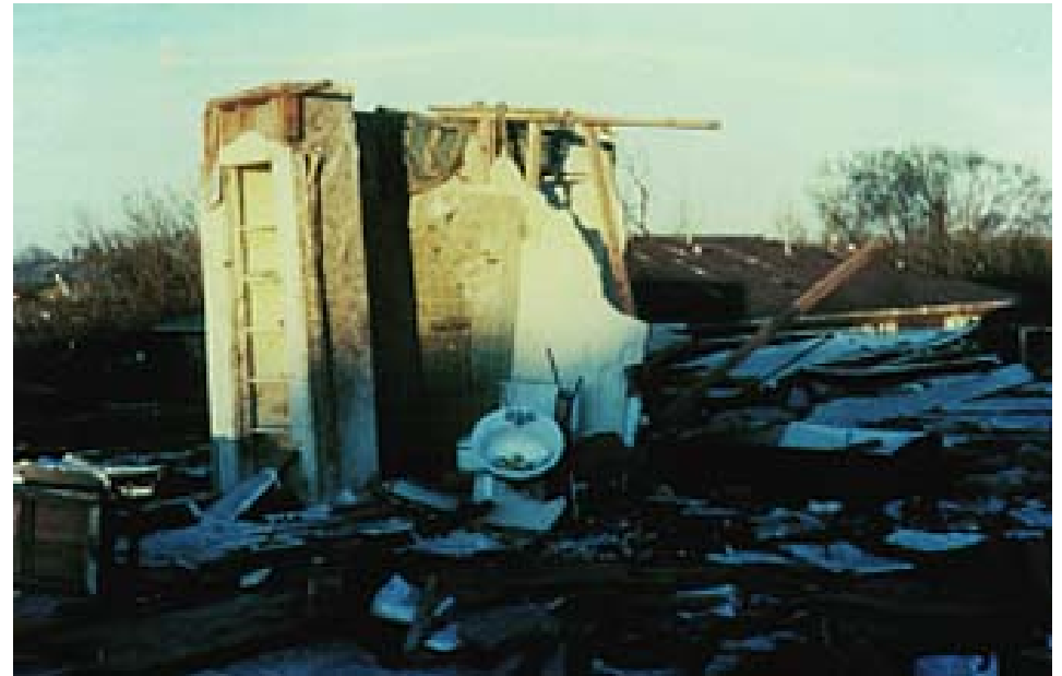
Interior bathroom was all that was left standing of this house:
