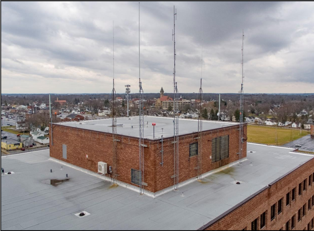
View of the RF devices from the Southwest corner (from the West side)
