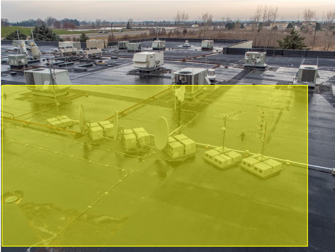
View of RF Devices and the spatial RF hazard area.
