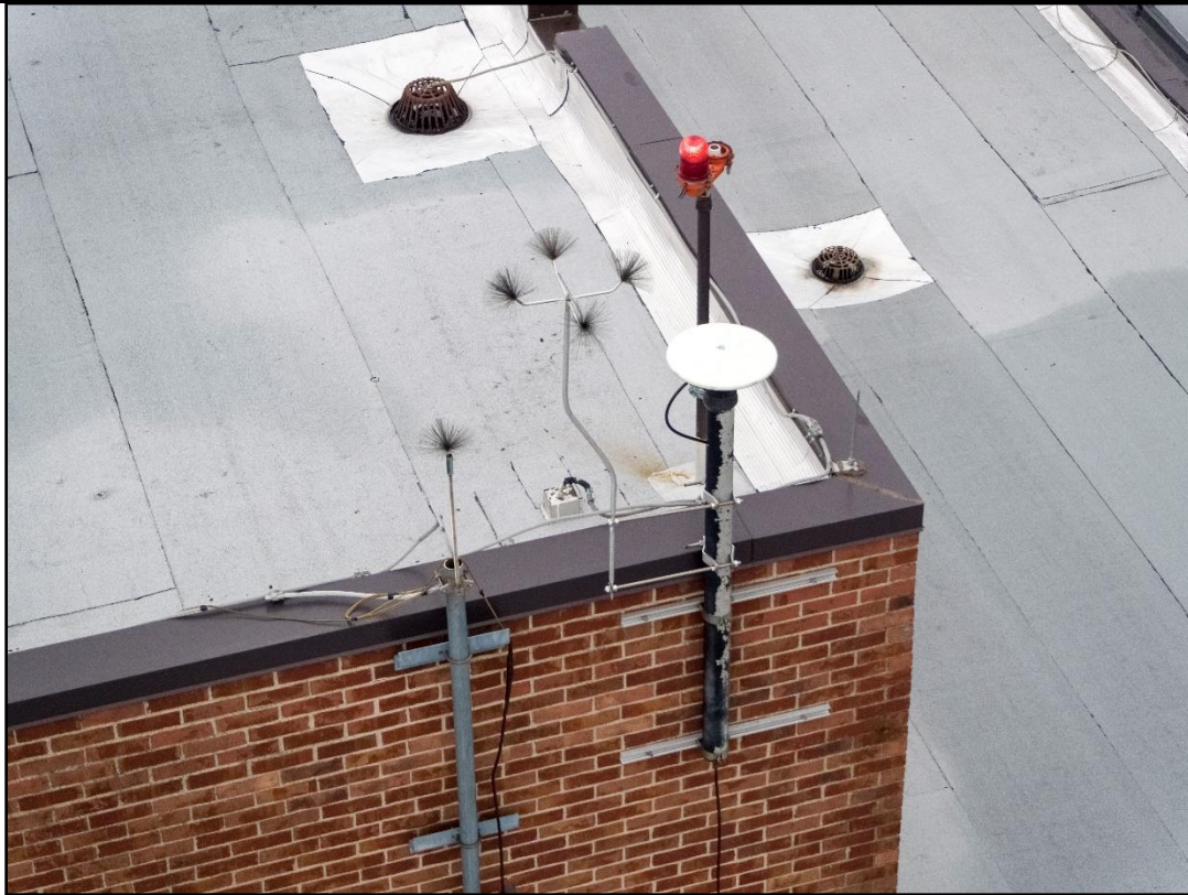
View of RF devices from the South side (from the Southwest corner)
