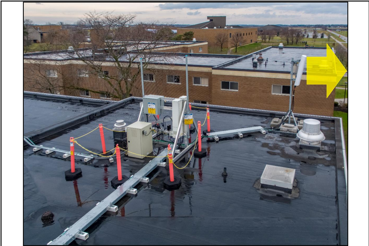
View from the South-end of the RF sources and directional RF energy.
