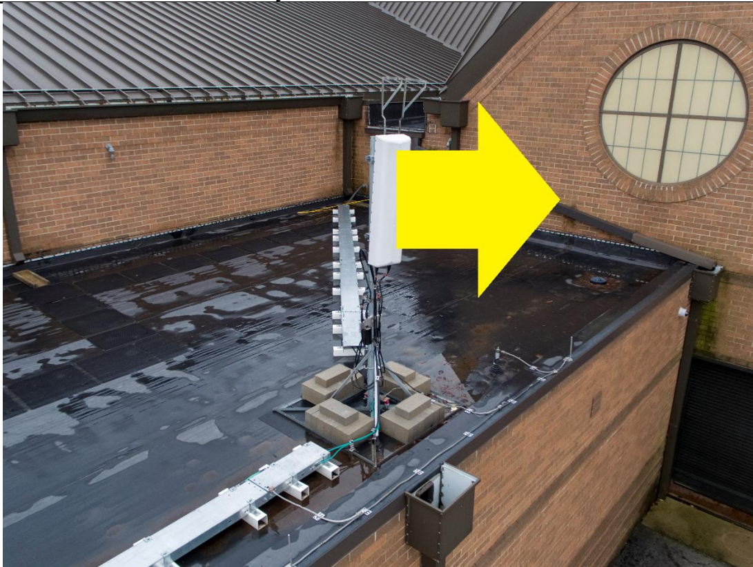
RF device furthest south on the rooftop and directional RF energy.
