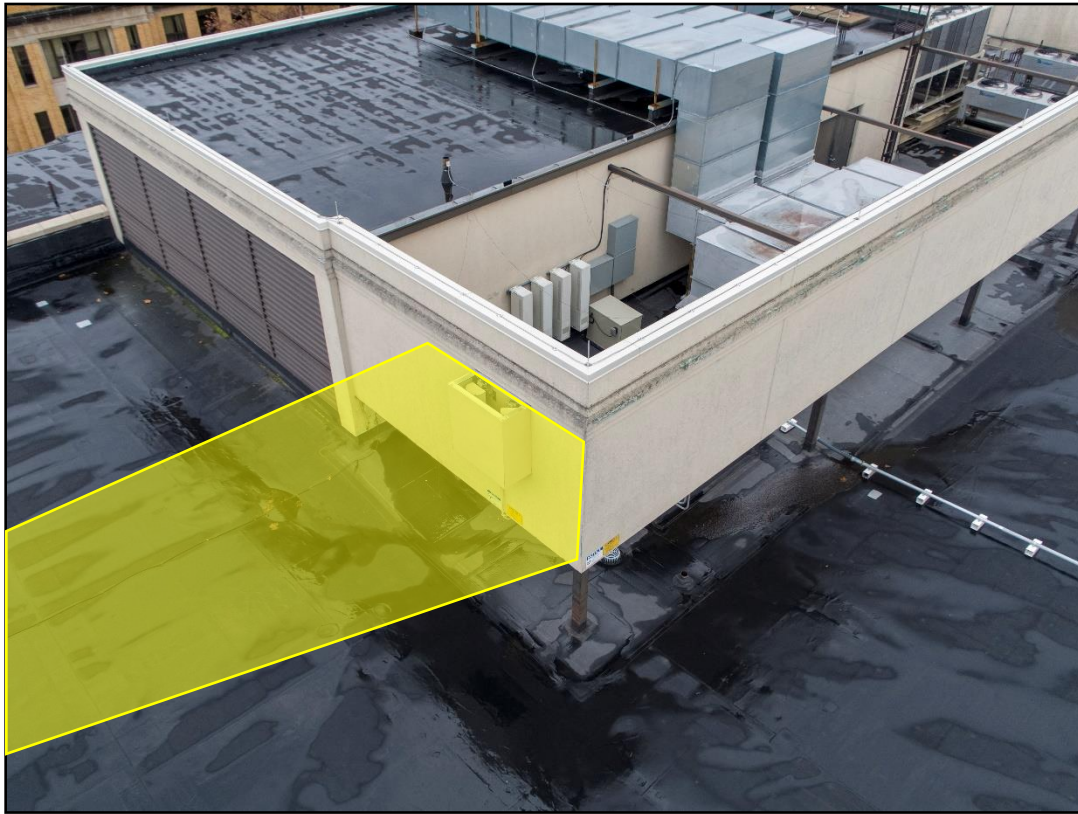
View from the West of the RF source (RF source is North facing)
