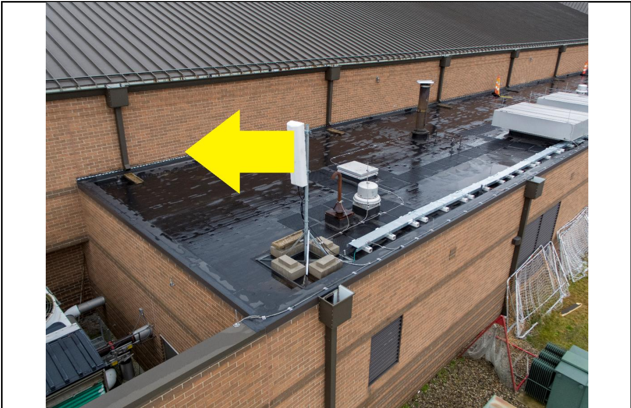
RF device furthest north on the rooftop and directional RF energy.
