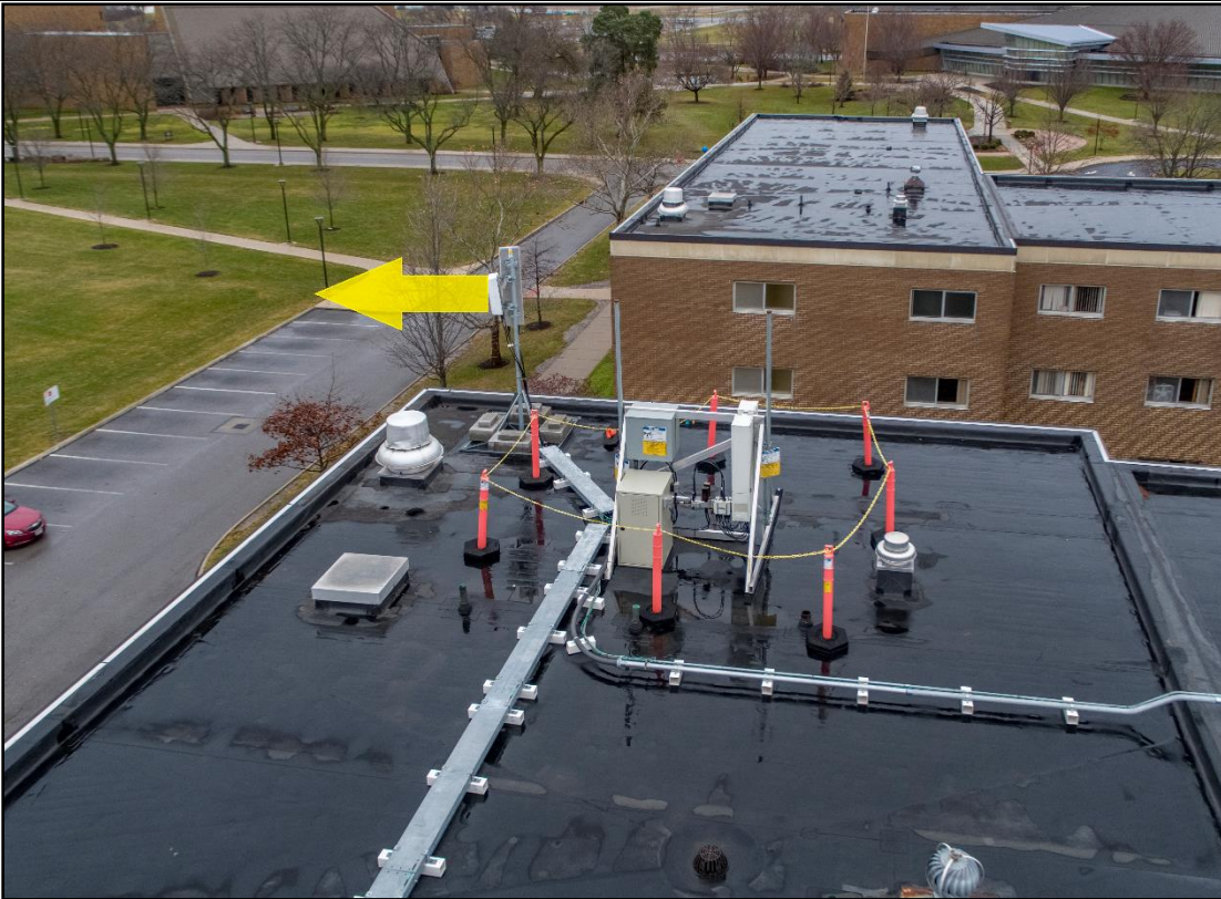
View of RF source at Kreisler- Ashley Hall and the directional RF energy.
